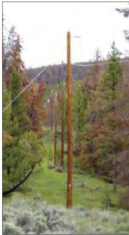
Many of Mountain Parks Electric's distribution lines are threatened by dead and dying lodgepole pine trees that can fall on conductor, knock out power and possibly cause a major wildfire. Photo by Les Shankland of Mountain Parks Electric.
